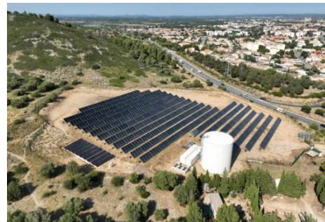
Figure 6. Aerial view of NARBOSOL solar thermal plant in Narbonne (France)
