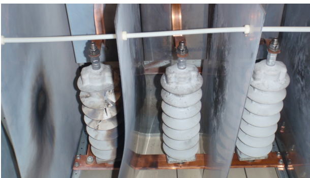
Figure 4: Broken surge arrester to the far-left
