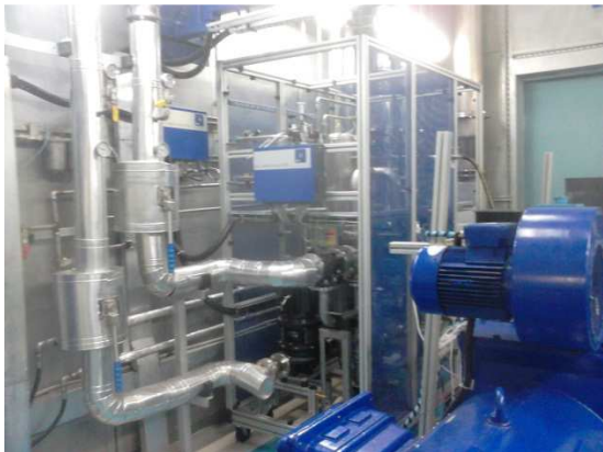
Figure 4: Thermal shock rig (test cell side) with test bed (blue), routing valves and pipes on the left.
