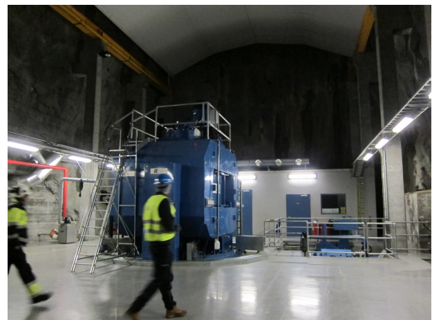
Figure 6: Grunnåi power station with its generator
