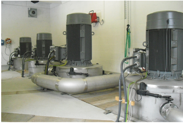
Figure 7: The four generator units in Sagbekken 2 and 3
