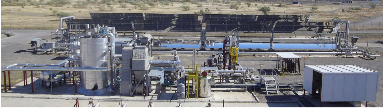
Figure 1. CIEMAT-PSA molten salt testing facility.
