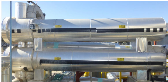
Figure 2. Thermal oil - molten salt heat exchanger.
