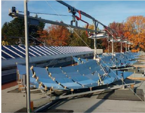
Figure 3. NRC concentrating mirror and flat panel solar PV systems
