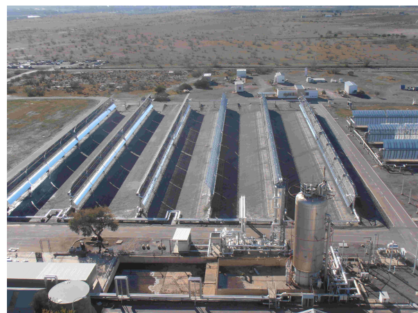
Figure 1. The TCP100 PTC solar research facility at Plataforma Solar de Almería (PSA-CIEMAT), (Pérez et al. 2018).
