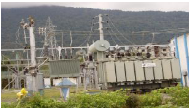
Fig [1]: A power transformer in a 63/20 KV substation, West of Mazandaran
