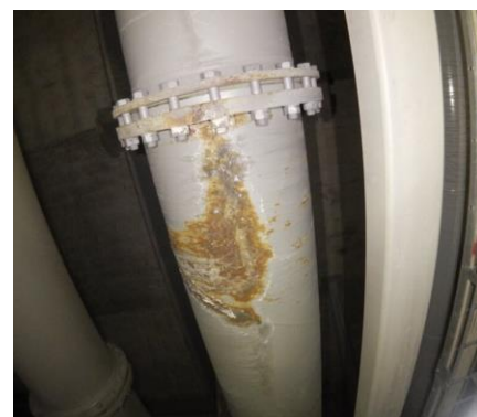
Figure 11. Flotation area, rusty pipe.
