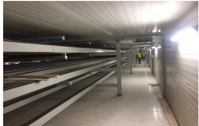
Figure 2. The dryer in the coating plant, showing the upper, middle and lower floors in one drying zone. Note the air ducts close to the ceiling, which supply the drying air to all levels.
