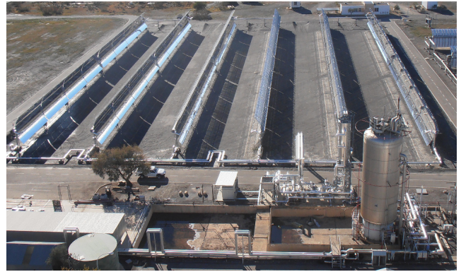
Fig. 1. Top view of the TCP-100 field at Plataforma Solar de Almería (PSA-CIEMAT). The three loops are shown, with two PTCs in each of them, numbered from 1 (rightmost) to 6 (leftmost). The first loop is formed by the connected pair 1-2 (right loop), the second loop by 3-4 (center loop) and the third by 5-6 (left loop).
